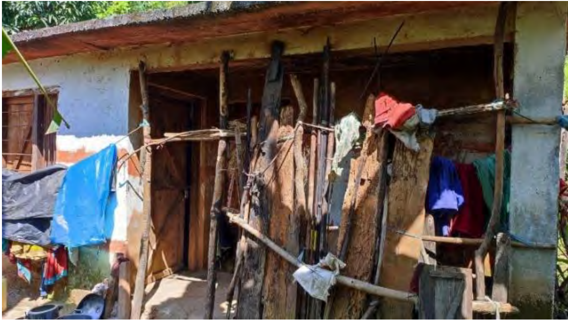
Condition of Raji houses in Kuta Chorani
