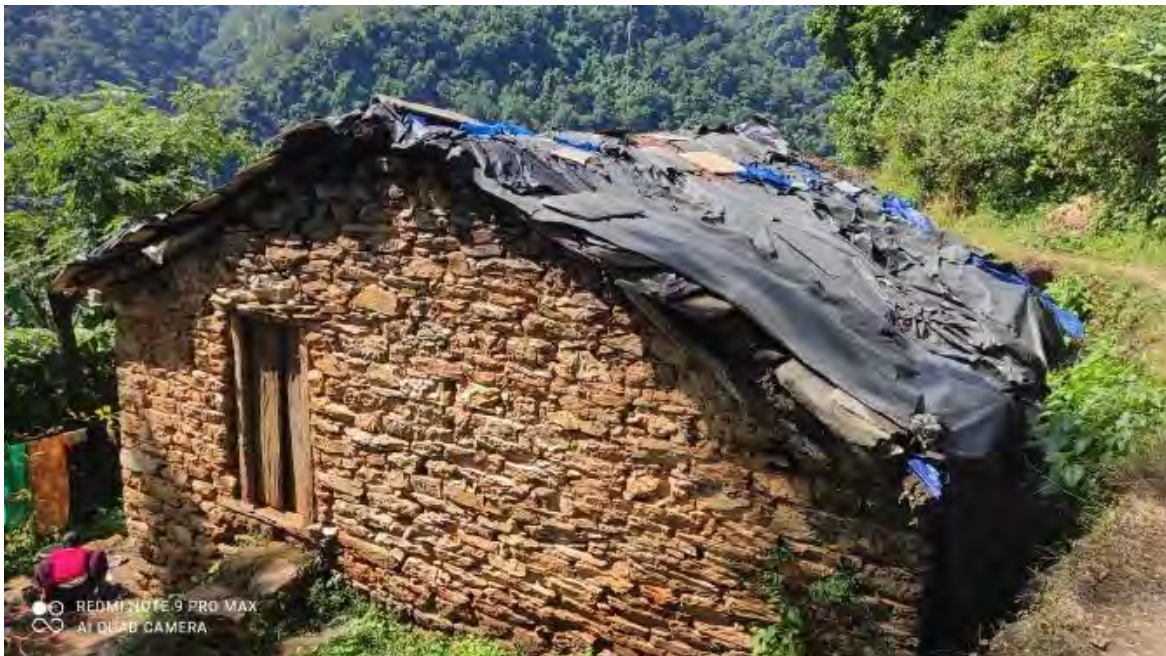
Condition of Raji houses in Kuta Chorani
